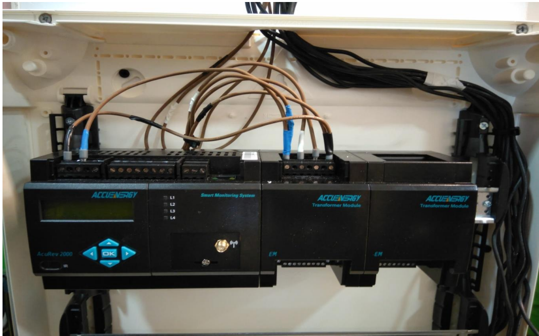
Figure 27: Photo showing the wiring of the voltage reference and power supply lines of the Accuenergy AcuREV 2020 meter deployed at the ICAEN pilot site
