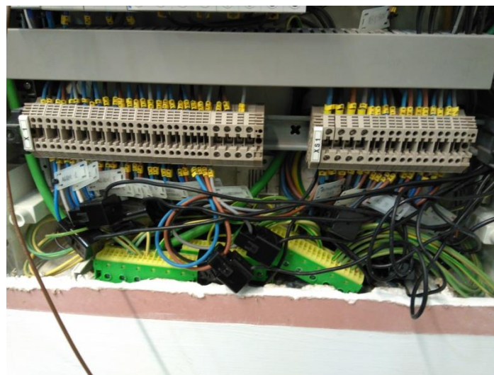
Figure 32: Photo showing the current transformers heads clamped to the electrical circuits
