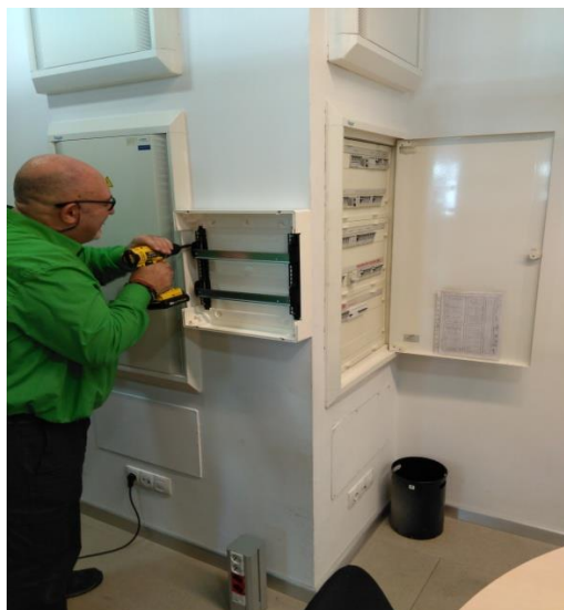
Figure 28: Electrician adding an enclosure to locate the meter outside of the electrical panel compartment
